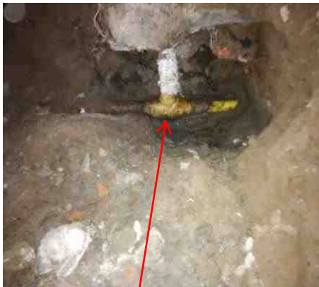
Fig 4- Illegal pipeline connection using T
