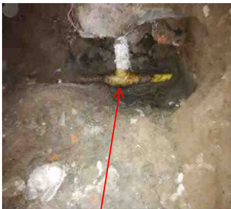
Fig 4- Illegal pipeline connection using T
