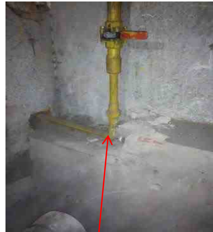
Fig 5- By passed meter pipeline concealed under wall
