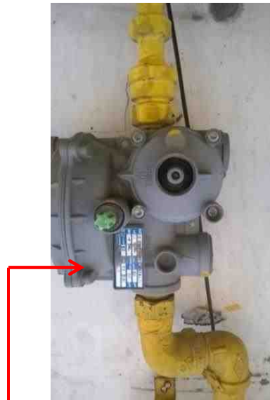
Fig 6 - Leakage point. (regulator reduces pressure from 4 bar to 21 mbar)
